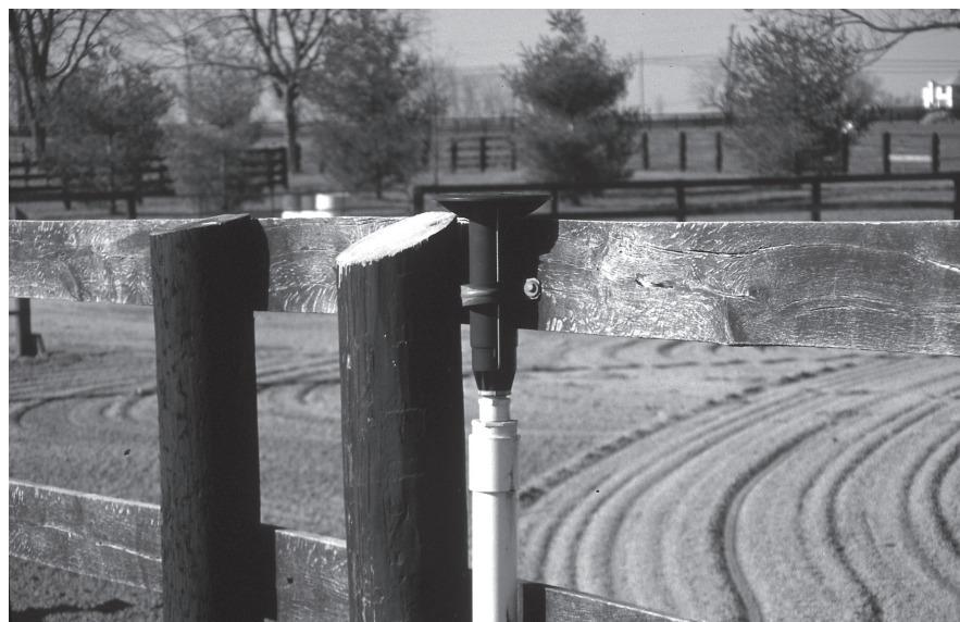
Figure 6. Horticultural-type sprinklers can be used in indoor and outdoor arenas to automate the surface-watering process.
